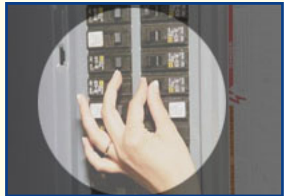
2. During a power outage with GenerLink™ simply turn off the breakers in your home's circuit panel.
