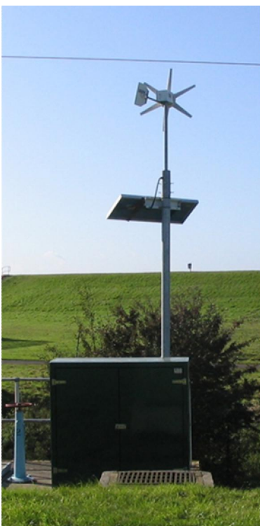
A low energy remote power site where a grid connection would otherwise cost thousands of pounds
